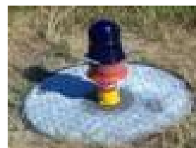
Taxiway Edge Lights
