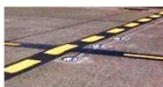
Taxiway Intersection Lines
