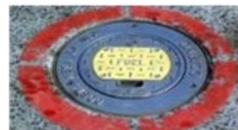
Hydrant Fueling Pit
