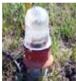
Runway Edge Lights
